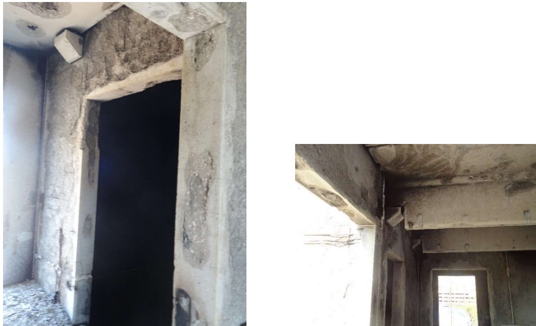
FIGURE 4.6: (a) Exposed reinforcement. (b) Corbel supporting double T joist.
