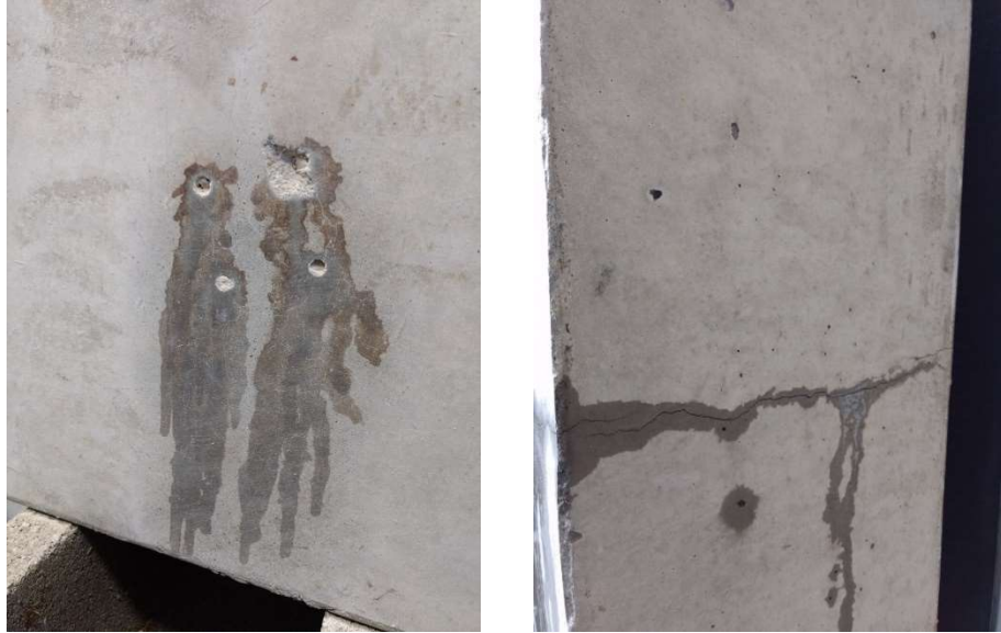
FIGURE 4.43: Leakage in specimen N2: (a) Plastic reinforcement chairs. (b) Horizontal cracking.
