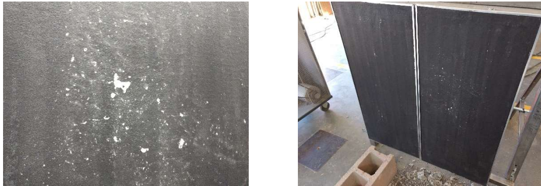
FIGURE 4.73: Raymax 2030 panel damage from spalling.
