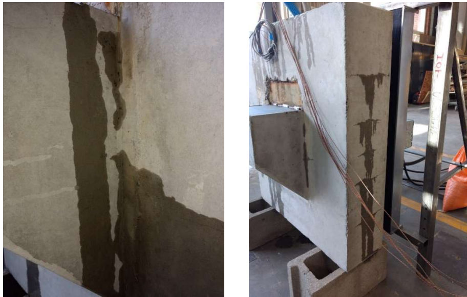
FIGURE 4.84: (a) Isolated corbel cracking, N2. (b) Isolated corbel cracking, N5.
