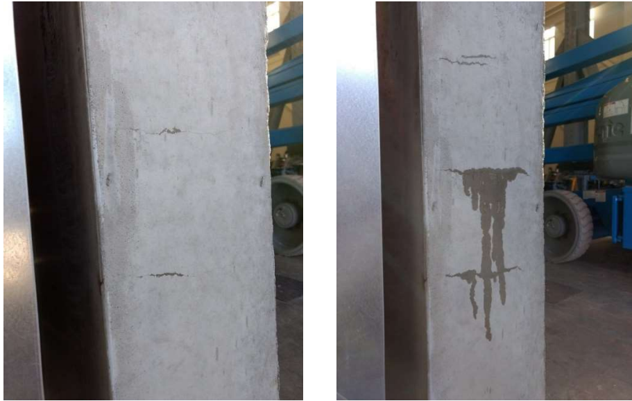
FIGURE 4.58: Specimen N5: Formation of tiered cracking.
