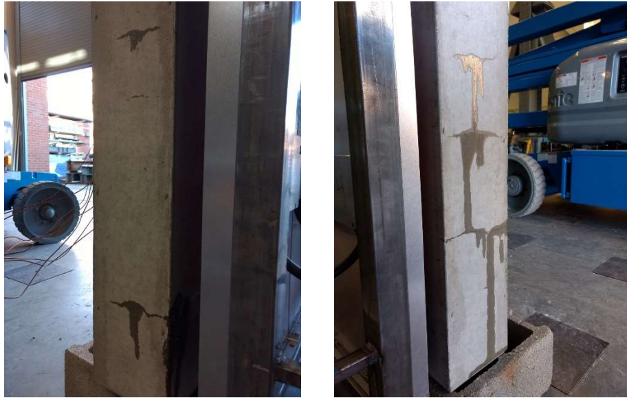
FIGURE 4.62: Specimen N6: Formation of tiered cracking.
