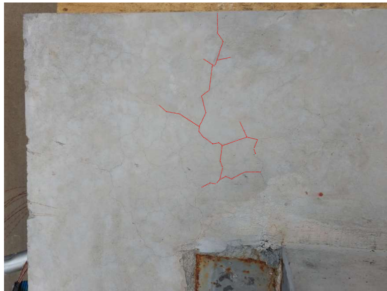
FIGURE 4.46: Specimen N2: Map cracking on corbel face after experimental test.
