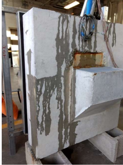
FIGURE 4.83: Full test duration cracking and leakage, N5.
