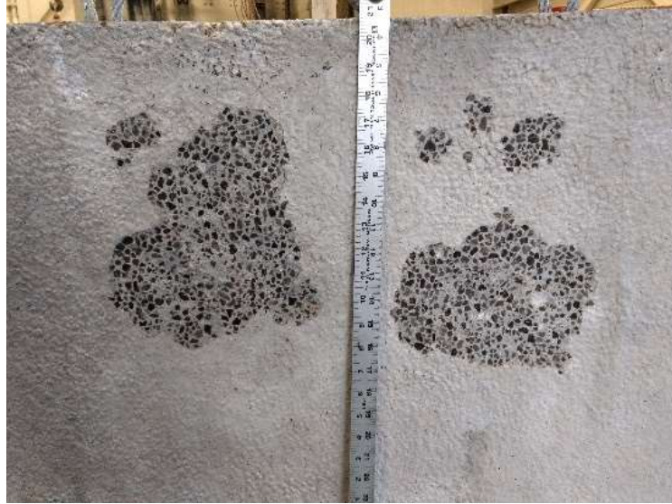
FIGURE 4.68: Spalling damage of specimen L8.
