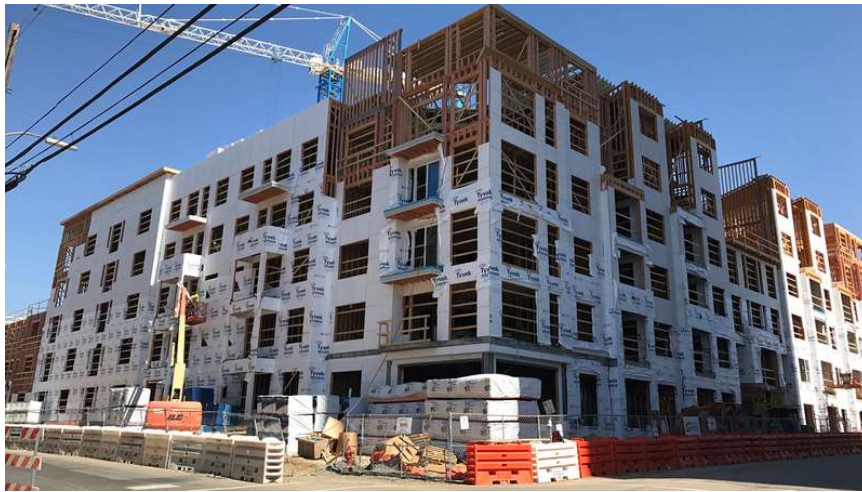
FIGURE 4.1: Pre fire apartment building Raleigh, NC (Wtvd, 2017).
