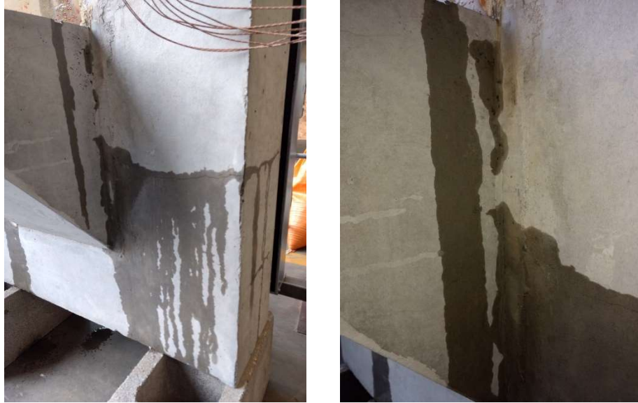
FIGURE 4.45: Specimen N2: Significant moisture leakage across specimen.
