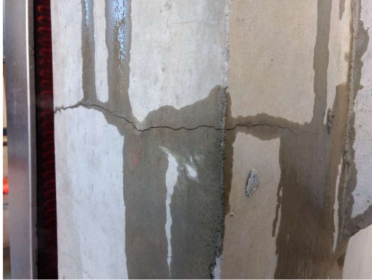
FIGURE 4.64: Specimen N6: Significant moisture leakage across specimen.
