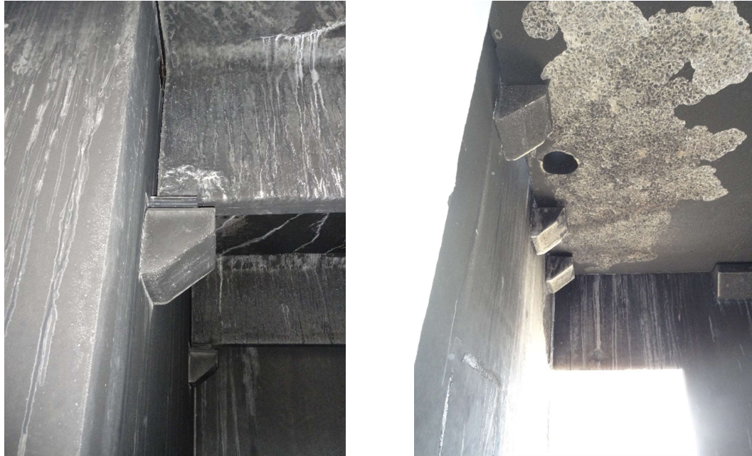
FIGURE 4.5: (a) Corbel and exposed bearing plates. (b) Ceiling spalling.
