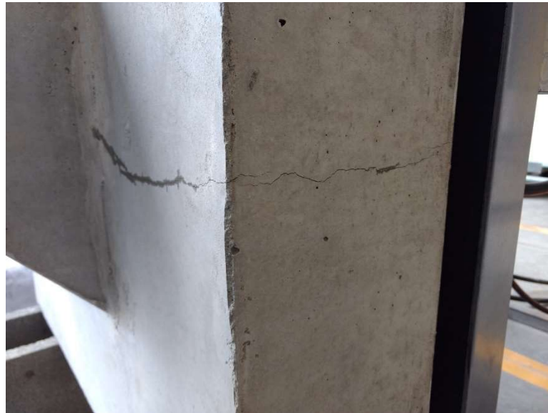
FIGURE 4.44: Specimen N2: Initial cracking and leakage, corner to front face.
