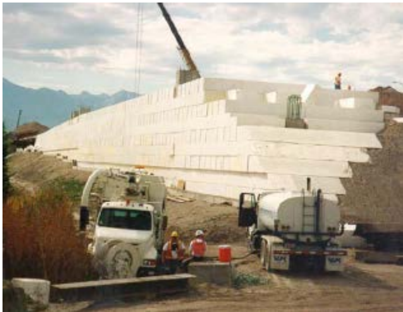
Figure 2.21: Typical EPS Geofoam embankment construction on the I-15 reconstruction Project in Salt Lake City (Newman et al., 2010)
