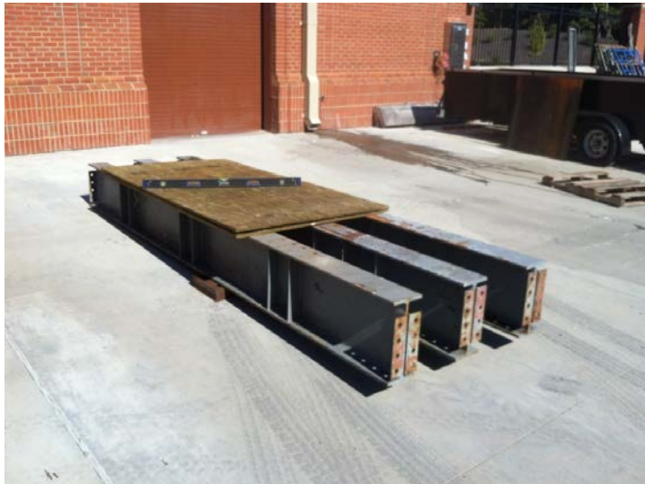
Figure 5.2: Photograph of the steel beam foundation constructed for the full-scale PET bale test specimen
