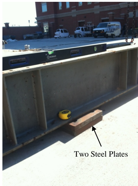
Figure 5.1: Photograph of a steel beam being leveled to serve as the foundation for the full-scale PET bale test specimen
