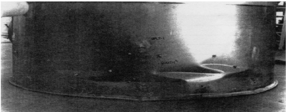
FIGURE 2.5: Diamond Shape Buckling of a Tank Wall
