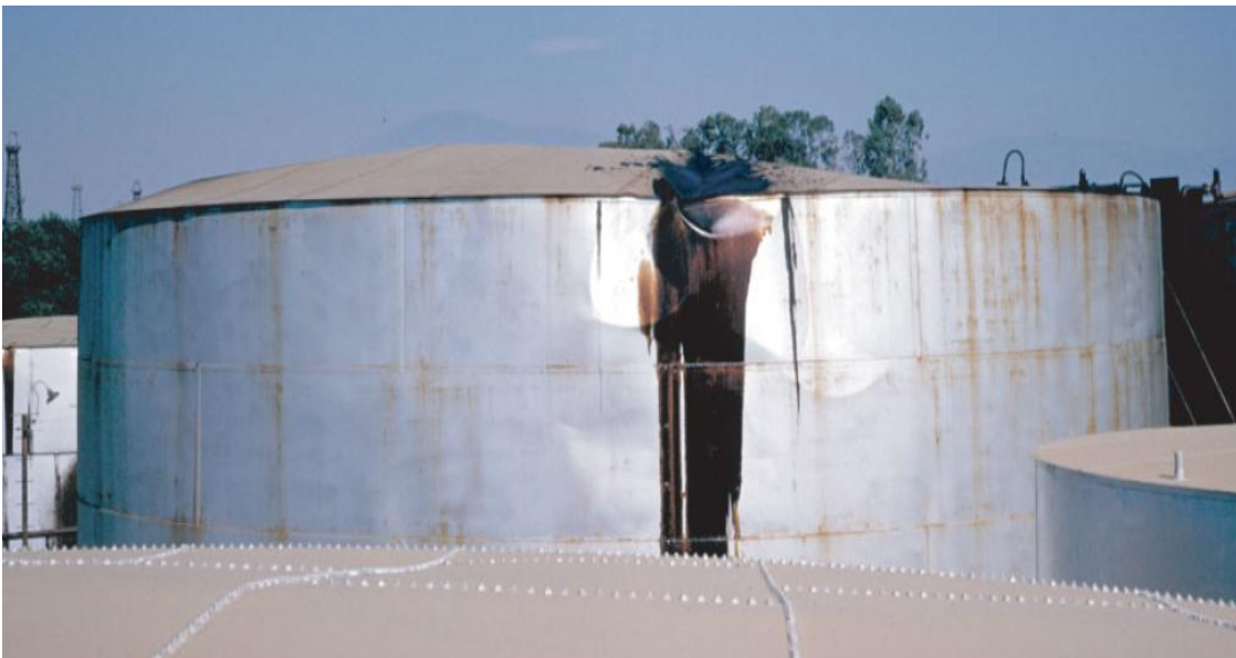
FIGURE 2.6: Damage to Roof and Wall Junction of Tank due to Convective Sloshing
