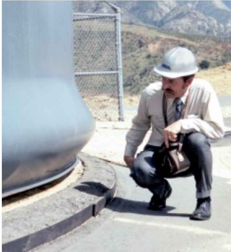
FIGURE 2.4: Elephant Foot Buckling of a Tank Wall
