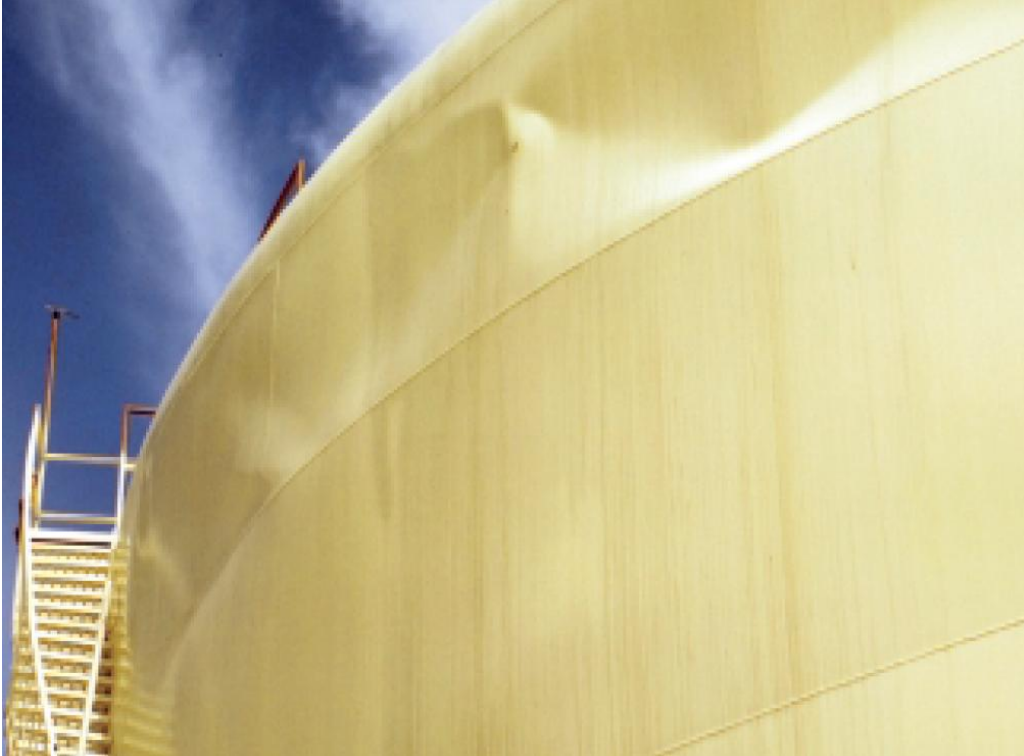
FIGURE 2.7: Damage to Upper Wall of Tank due to Convective Sloshing
