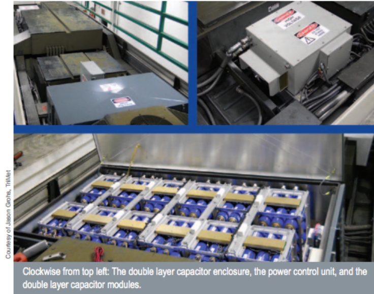
FIGURE 19: Roof-mounted capacitor stack, TriMet light rail fleet (U.S. DOT FTA, 2012)
