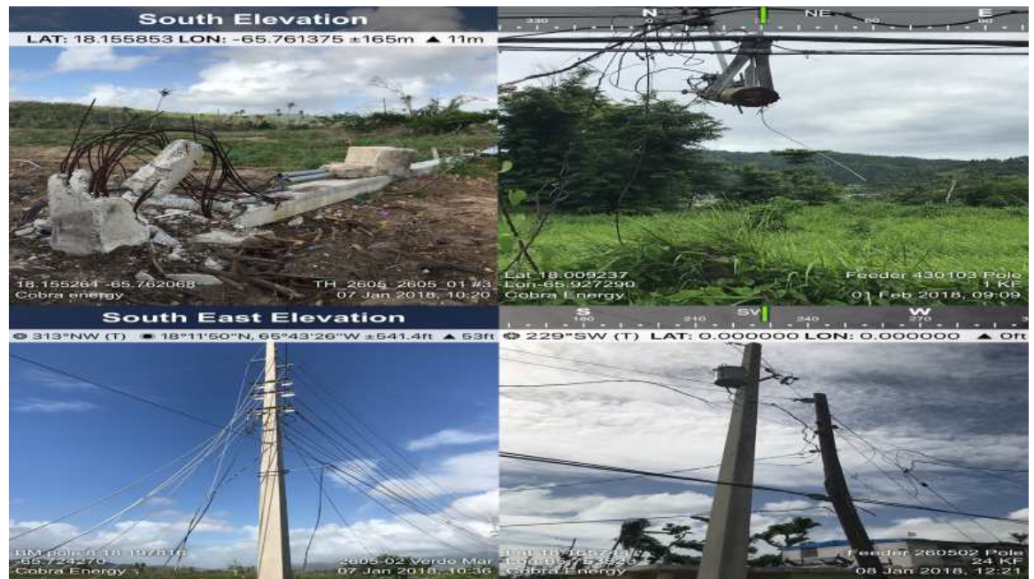
Figure 2.3: Various modes of damages to transmission structures (PREPA, 2018).
