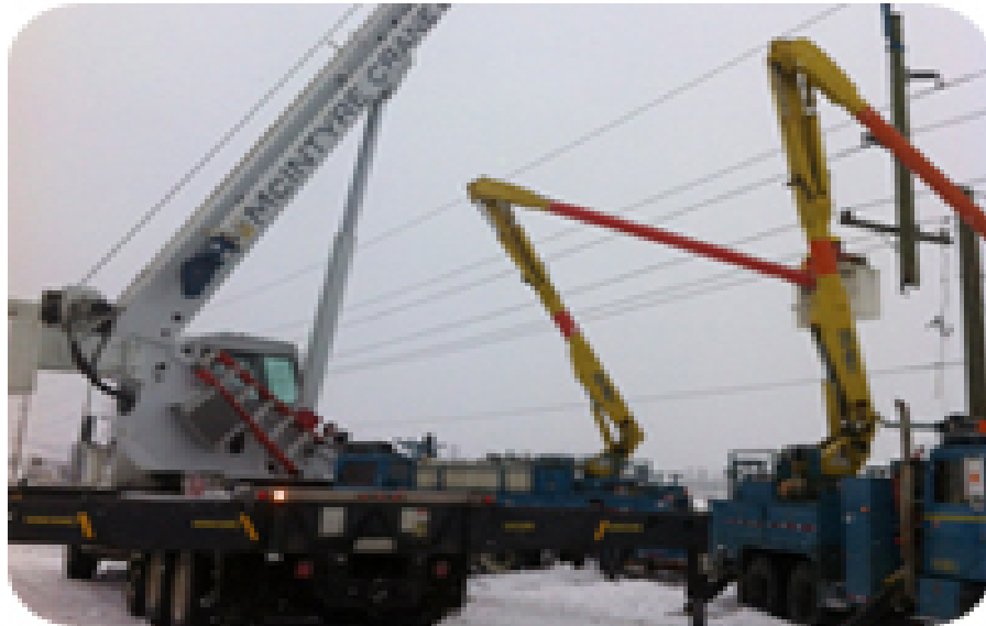
FIGURE 9: Crane in contact with power line Source: Crane accidents. (2012)
