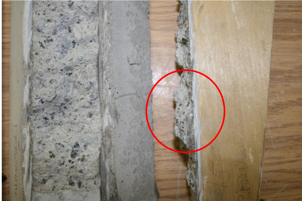
Figure 2.9 Deep Substrate Failure – FRACT27_T
