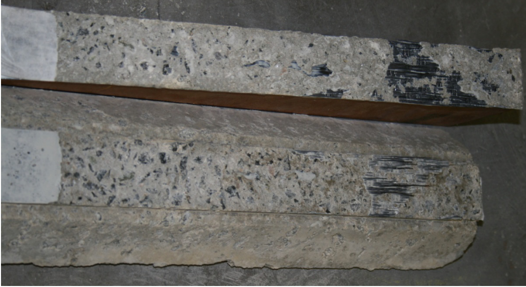
Figure B.10 Fatigue Failure – 200 Freeze/Thaw Cycles
